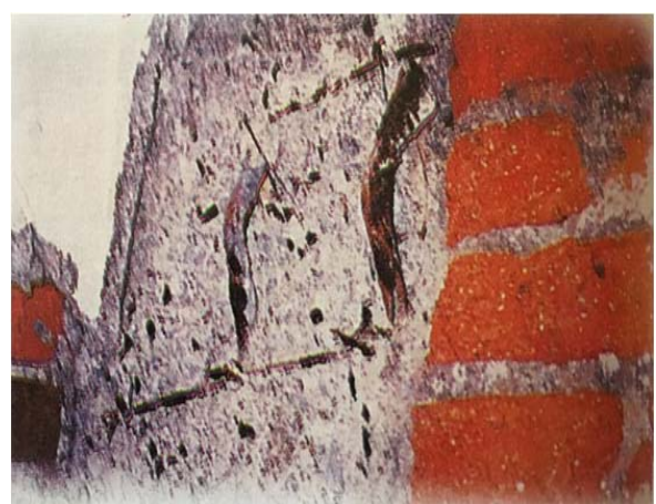
Figure 4: Several Distress in Building
