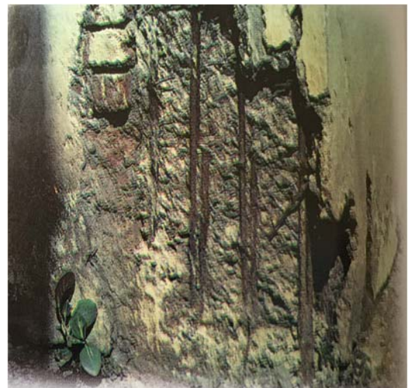
Figure 9: Corrosion of Steel in RCC Column
