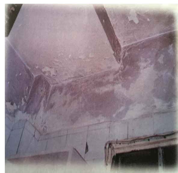
Figure 10: Leakages on Ceiling
